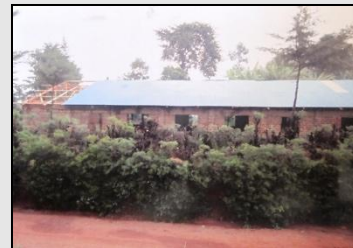
Moving the Vigetse Salvation Army church off school grounds opened up space for a school library
